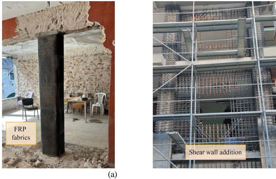
Figure 4. Examples for retrofitting of an RC building. (a) Member retrofitting, (b) System retrofitting
