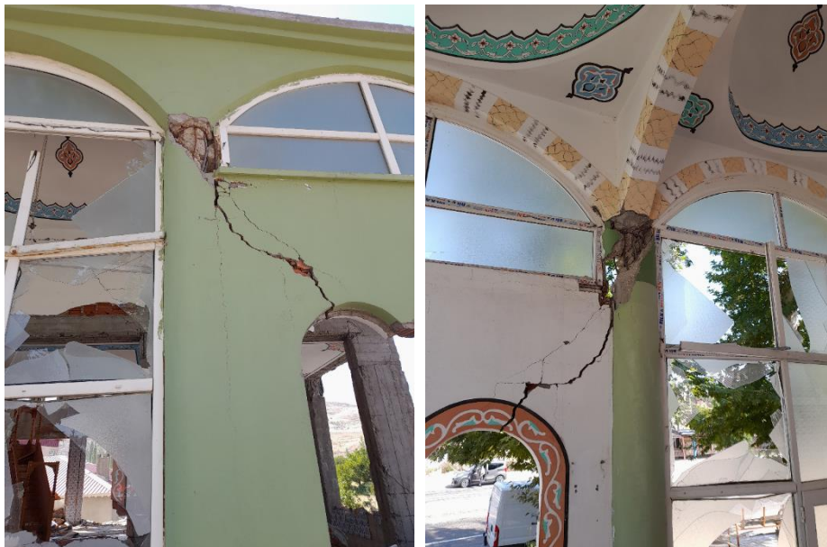
Figure 2. Short column damage due to infill wall
