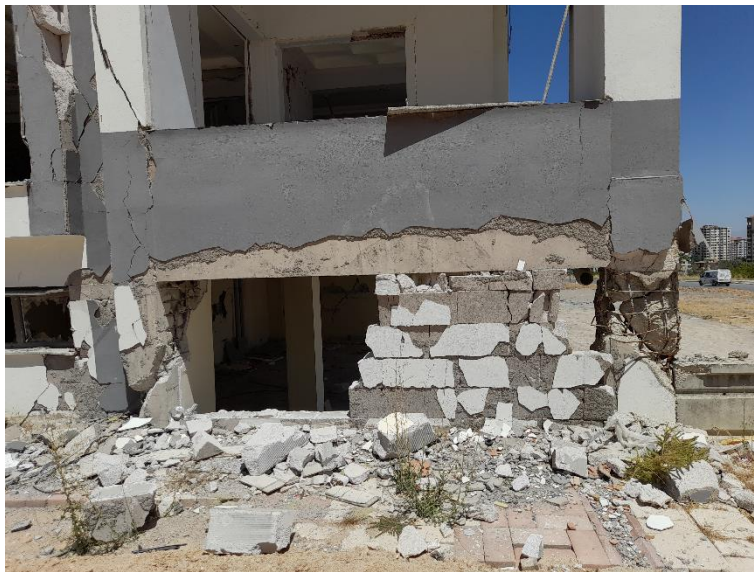
Figure 4. Short column damages due to basement and garden wall
