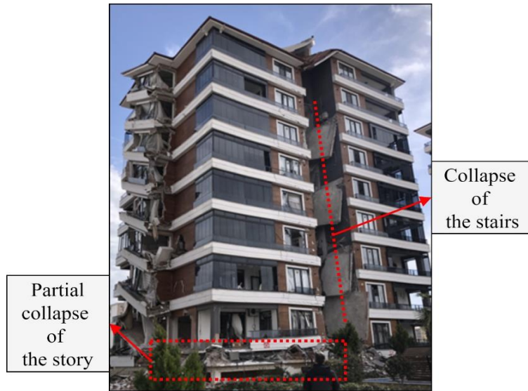
Figure 2. A mid-rise RC building to be urgently demolished.
