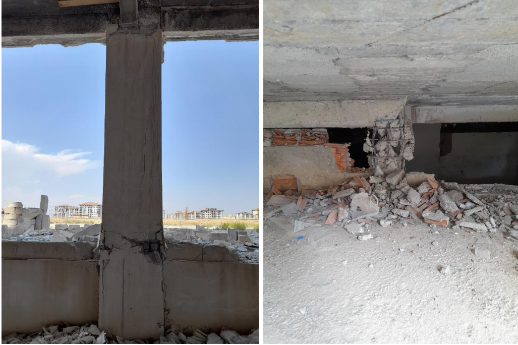
Figure 3. Short column damages because of basement
